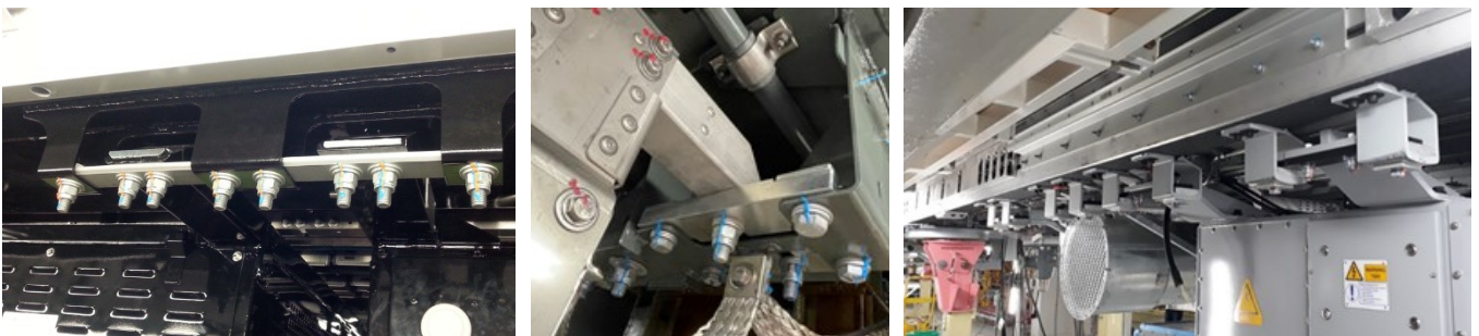
Figure 4: « Positive » equipment mounting on metro platform
